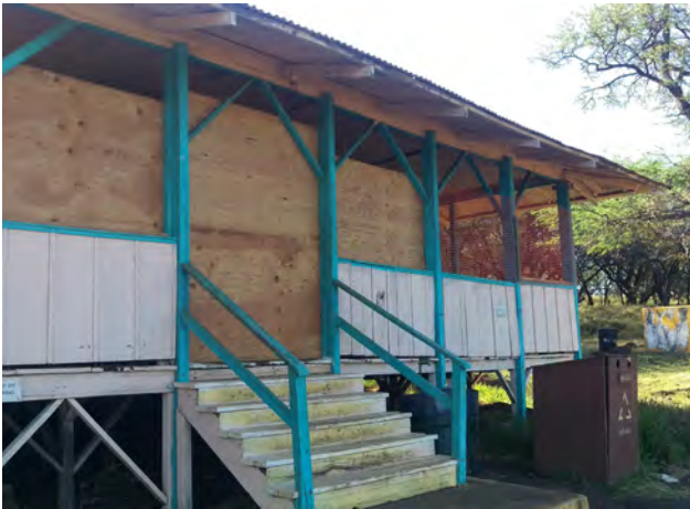
Condemned park pavilion
